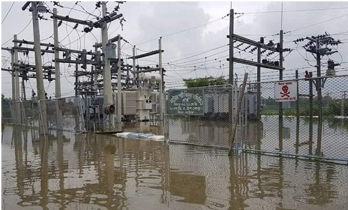
Figure 4: Substation flooded in Shingra, Natore
